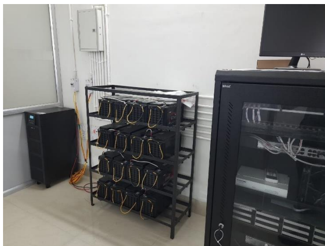
Pic 2: Centralized UPS
